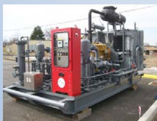
Natural Gas Compressors
